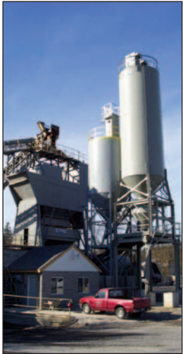
Dedicated slag silos are major capital investments, but they permit greater flexibility in delivering the best blend for each job.
