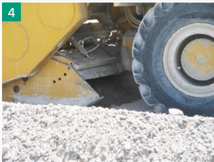
4 A second pass with the reclaimer to blend TerraCem into the soil
