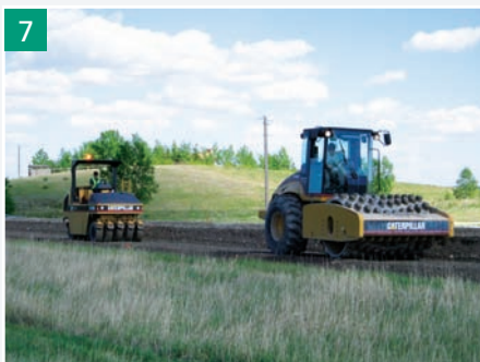
7 Vibratory pad-foot compactor followed by the pneumatic version to achieve a smooth top surface
