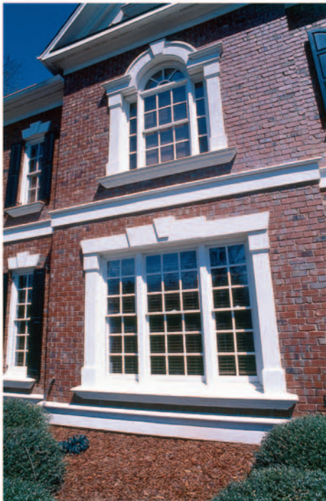
BOTTOM RIGHT Oversized window frames combine with glazed brick and matched masonry cement to produce a fresh take on a classic look.
