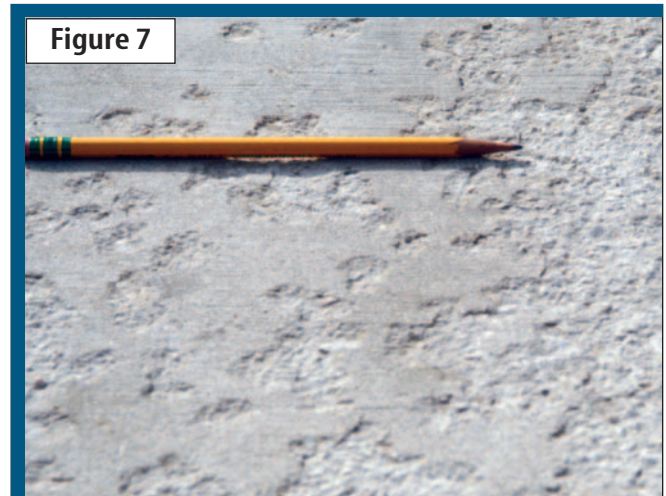
When the hydraulic pressure of water's freeze-thaw in the concrete exceeds the material's tensile strength, scaling can result in the absence of entrained air voids.
