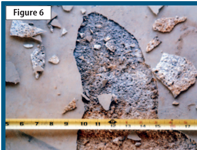
Unightly delaminations, like the one in the photo above, can be minimized through avoiding the use of concrete with excessive slump, air content, or fines.
