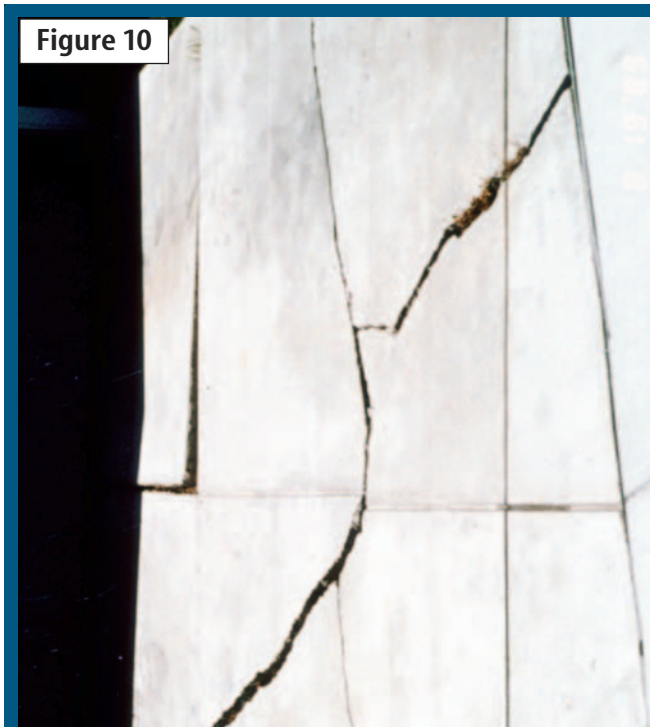
Settlement cracking occurs because slabs on grade cannot bridge a structurally deficient sub-base.
