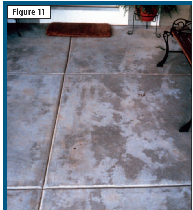
Concrete discoloration can occur due to numerous factors that must be considered to ensure the final aesthetic is the desired one.
